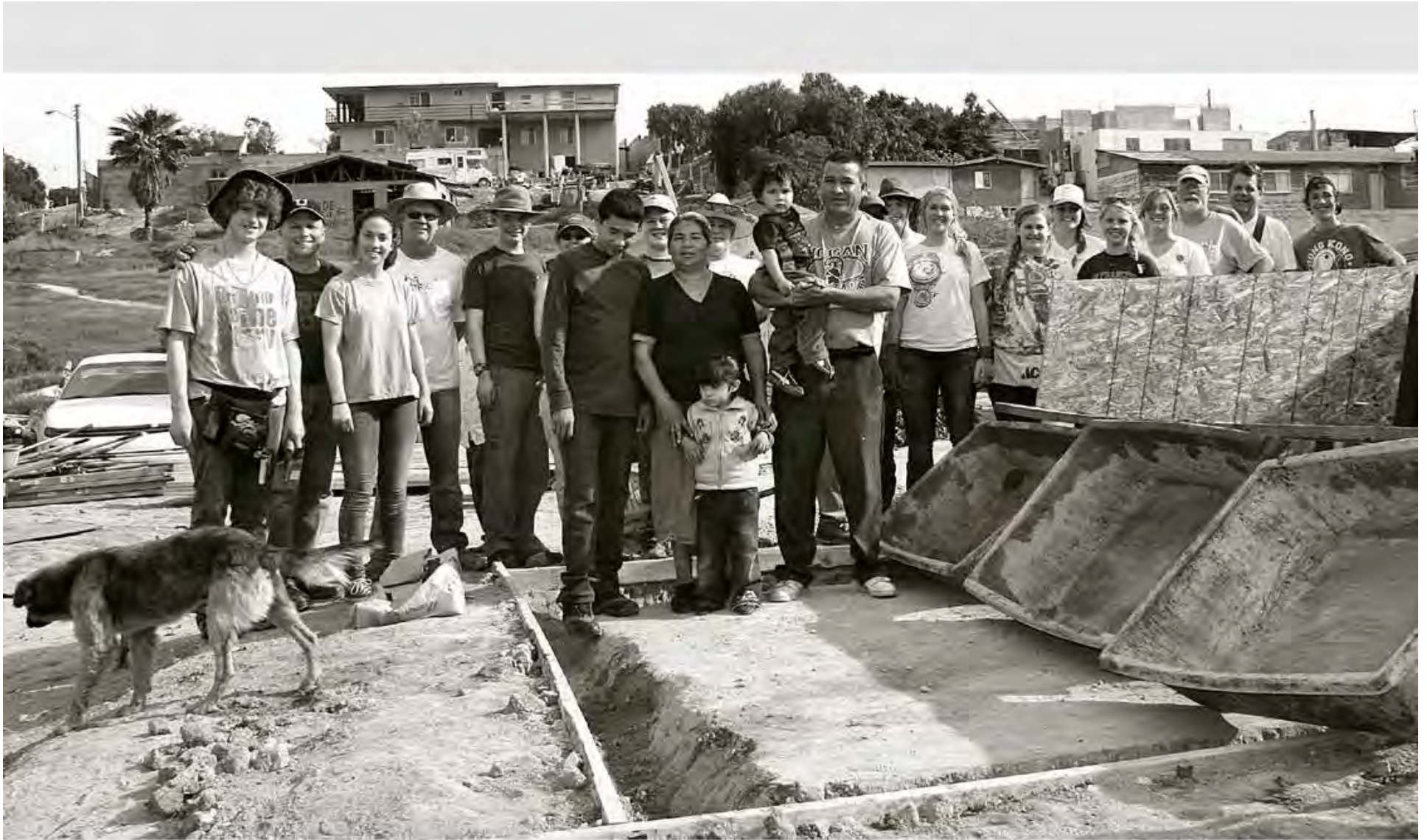
end of the first day one half of the foundation is laid and some walls are done
