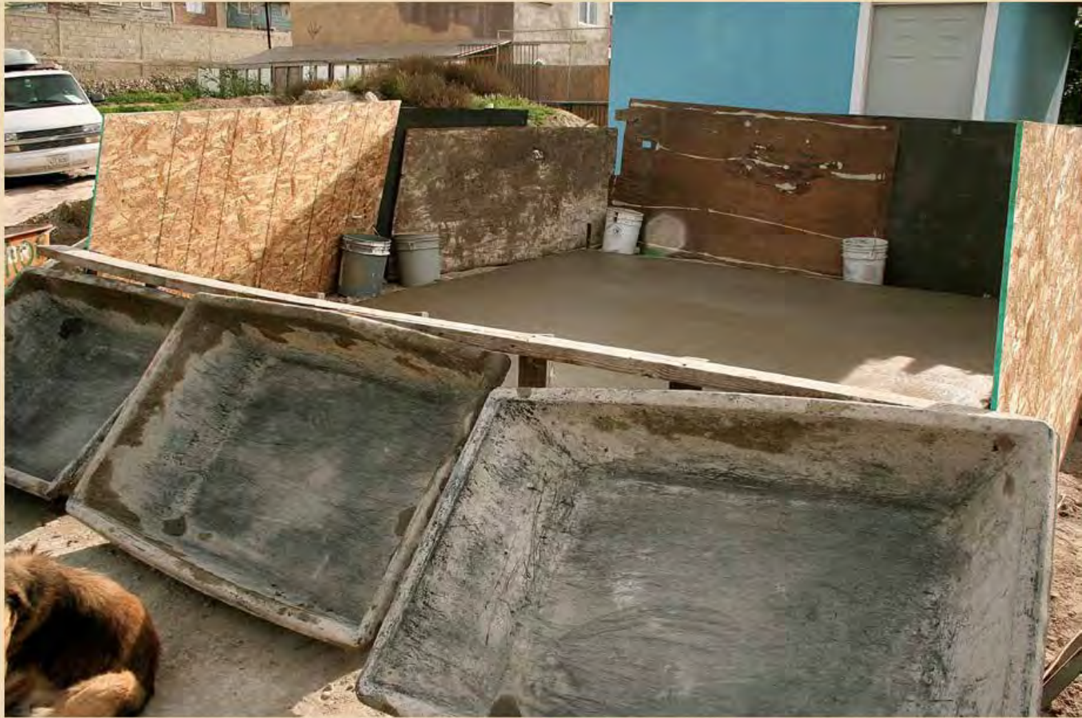
A barracade is built to protect the wet foundation from 10 dogs (and 2 children).
